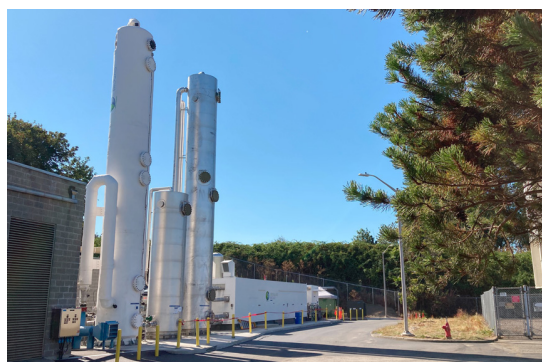
Cascade H 2 O installation
